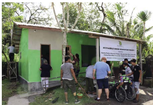
Many hands make light work – the Puspadi Bali community constructing an accessible house for people with physical disabilities.
